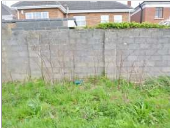
JK 1 : Last seasons Japanese Knotweed plant stems along the south eastern boundary wall – March 2019
