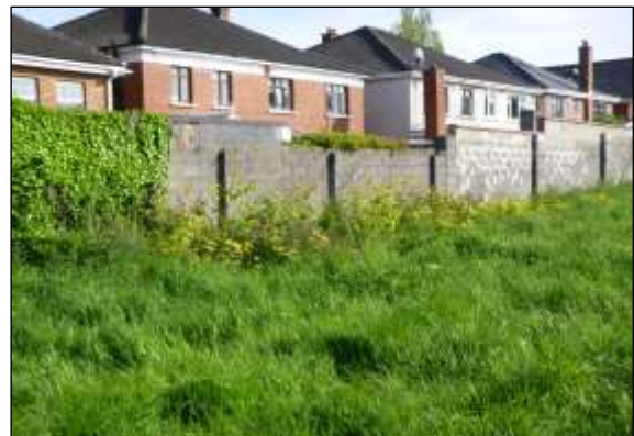
JK 1 : South eastern boundary wall, looking south. Emergent Japanese Knotweed showing good growth – May 2019
